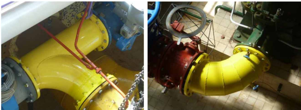
Figure 5 | New pipe elements in the discharge pipe of the pump house.
