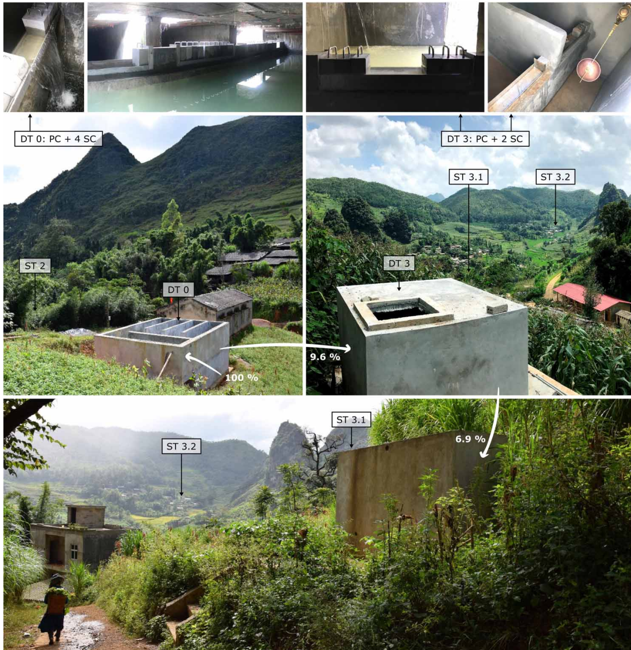
Figure 8 | DT 0 (under construction) with inside view (top left), DT 3 (under construction) with inside view (top right) and ST 3.1 in supply area West (bottom).
